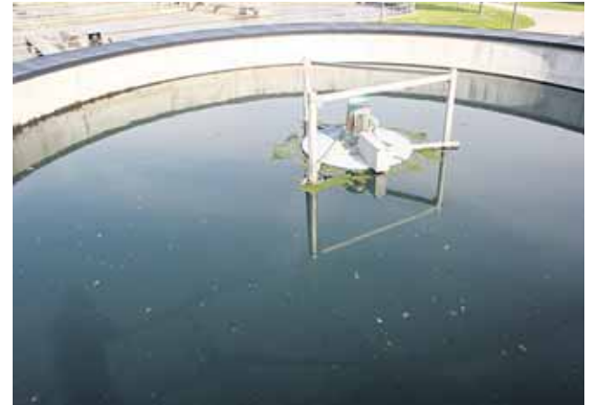
Digester tank ready for paddlefish. The aerator is in the center.
